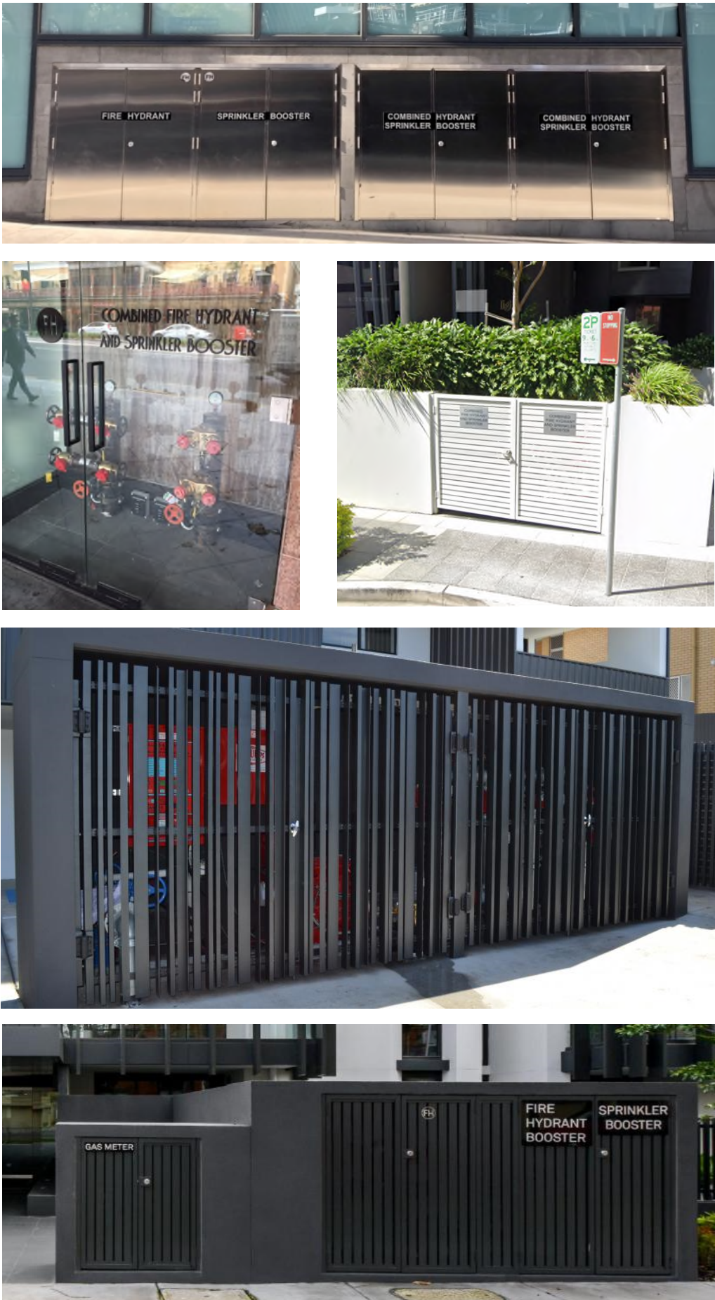
Figure 3. Examples of enclosed fire safety utilities
