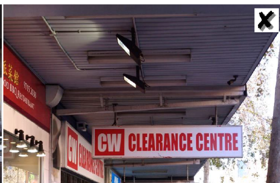
Exposed lights are not encouraged unless they are fitted and integrated within the fascia or consistent with the character of the building.
