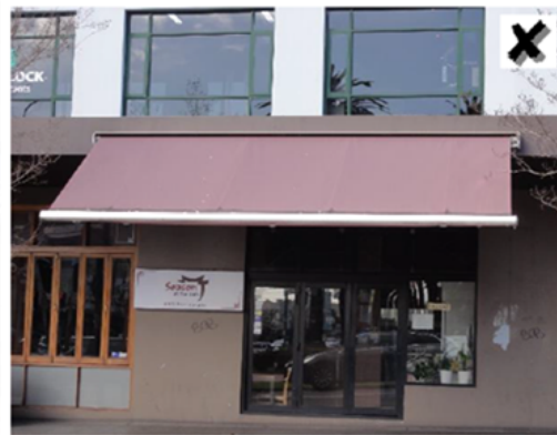
Awning extensions should not be fixed to the face of the awning fascia.
