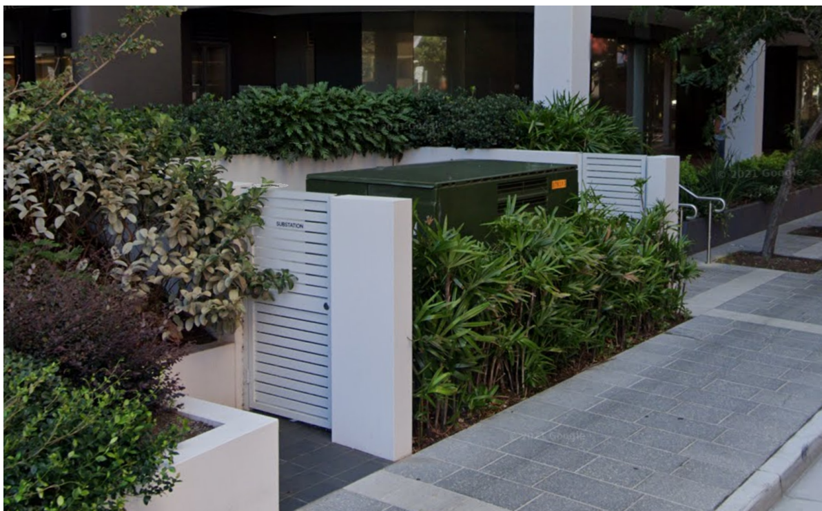
Figure 4. Example of a screened large power supply utility / substation
