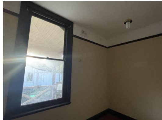
Figure 4.28 25 Woodside Avenue – bedroom window
